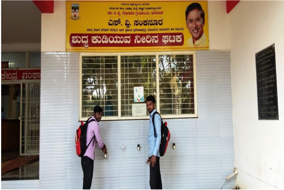
Reverse Osmosis (RO) drinking water facility for students and Staff at Dr.V.K.Gokak Library
